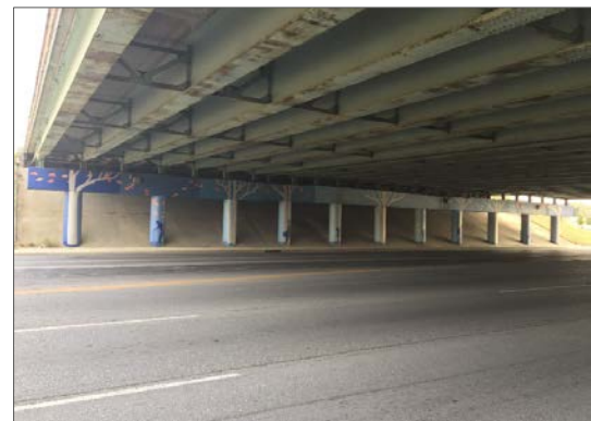
Many bridges in the project area show age-related wear such as rust and damage from leaking water. Photo Source: HNTB
